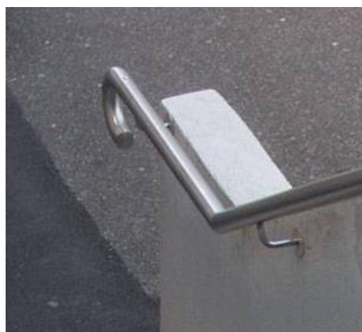
Figure 7.6: Compliant, rail extends beyond the stair
